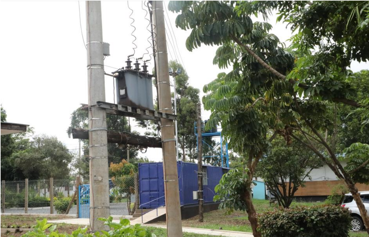
Figure 3: Current status of the proposed site showing the existing 50kVA transformer.
